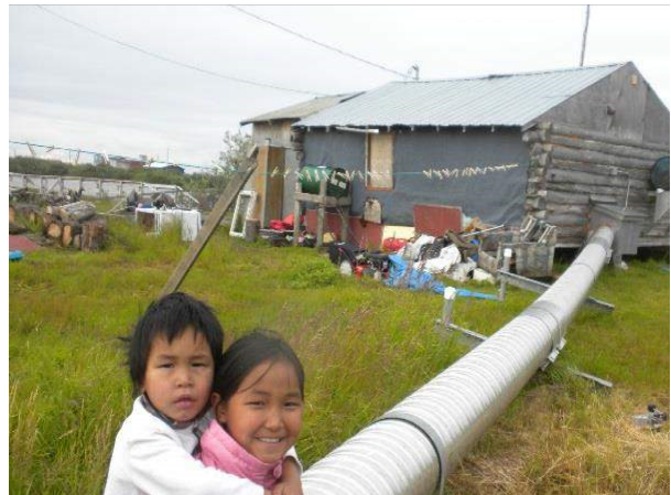
Figure 1: A collapsed service line due to permafrost thaw in Selawik. Reprinted from Brubaker, M. (2011) In M. Brubaker, P. Chavan, J. Berner, M. Black, & J. Warren (Eds.), Climate change in Selawik, Alaska: Strategies for community health , 2012 (p. 1). Alaska Native Tribal Health Consortium. Anchorage: ANTHC Center for Climate and Health. Copyright 2011 by Brubaker
